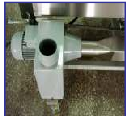
Figure 8. Ventilation fan outlet connection
